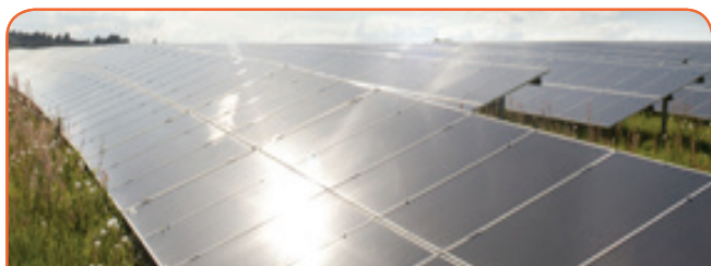
Photovoltaic solar cells produce usable electricity
