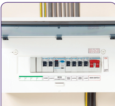
Circuit breakers are essential safety mechanisms, which protect an electrical circuit from current overload
